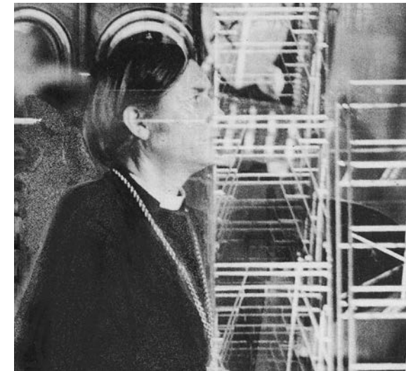
Repairing the Guastavino dome in the great crossing, 1973 photo credit: Beverly Hall
